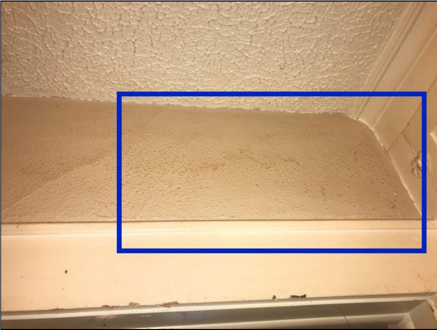
4.1 Item 2(Picture) prior moisture staining
