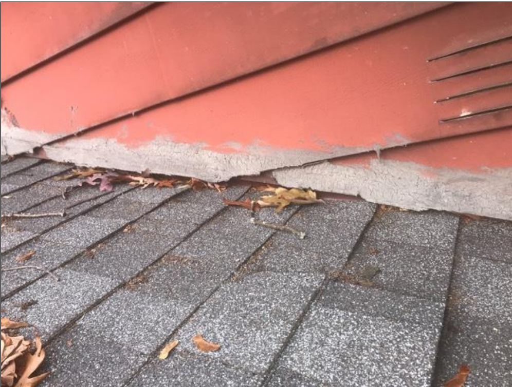
1.1 Item 1(Picture) flashing at gable not visible
