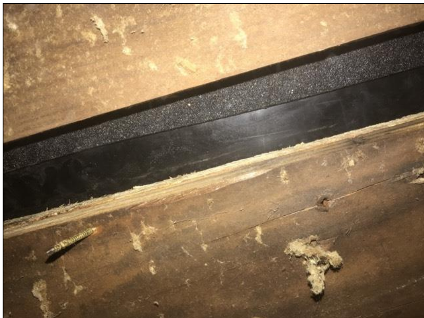
9.3 Item 1(Picture) shingle over intake vent
