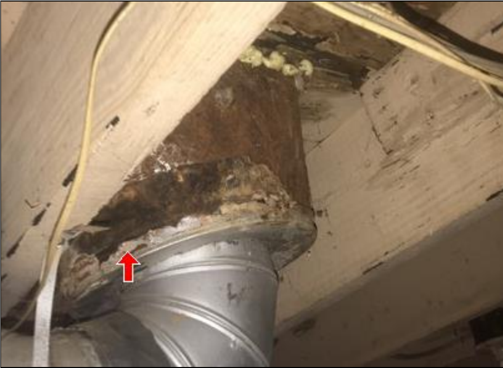
5.0 Item 8(Picture) basement hvac duct
