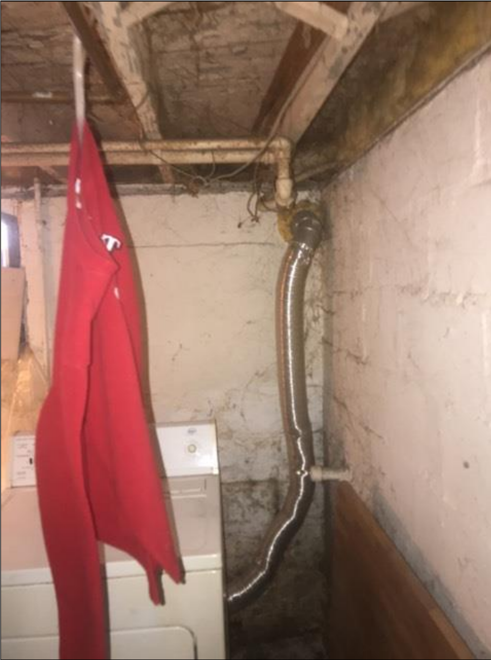
5.0 Item 4(Picture) water infiltration area
