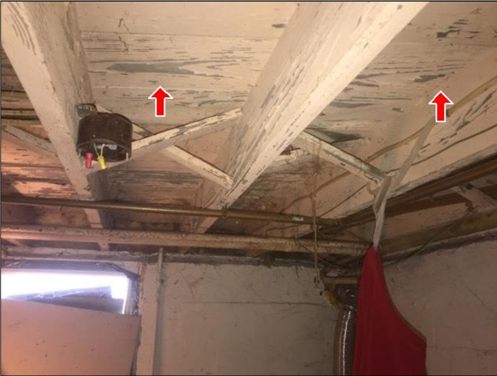
5.0 Item 3(Picture) peeling paint from condensation
