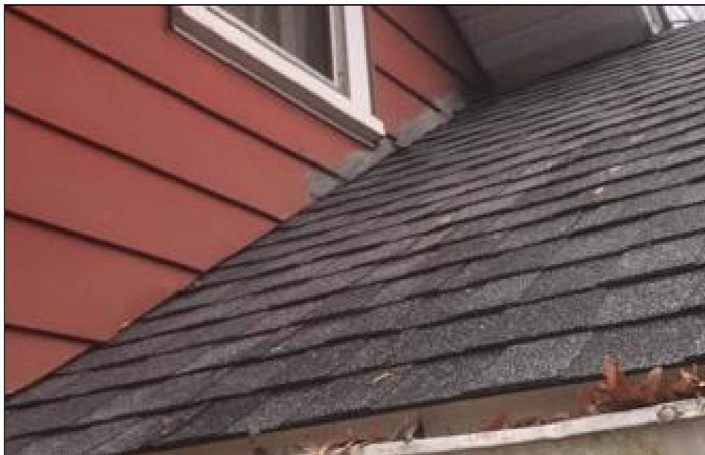
1.1 Item 2(Picture) no flashing observed
