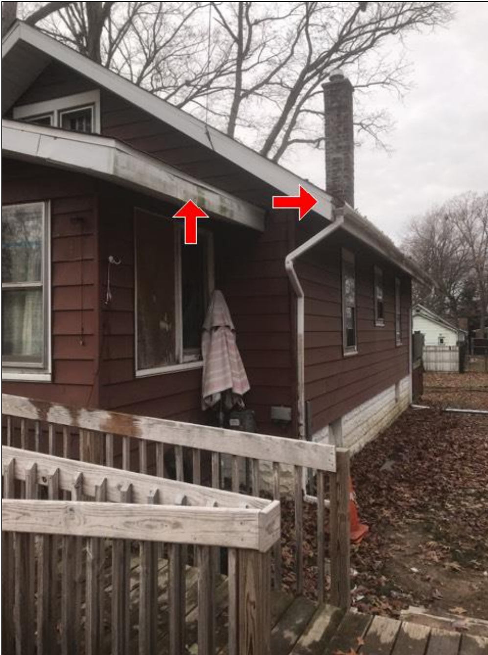
1.3 Item 1(Picture) gutter missing/damaged
