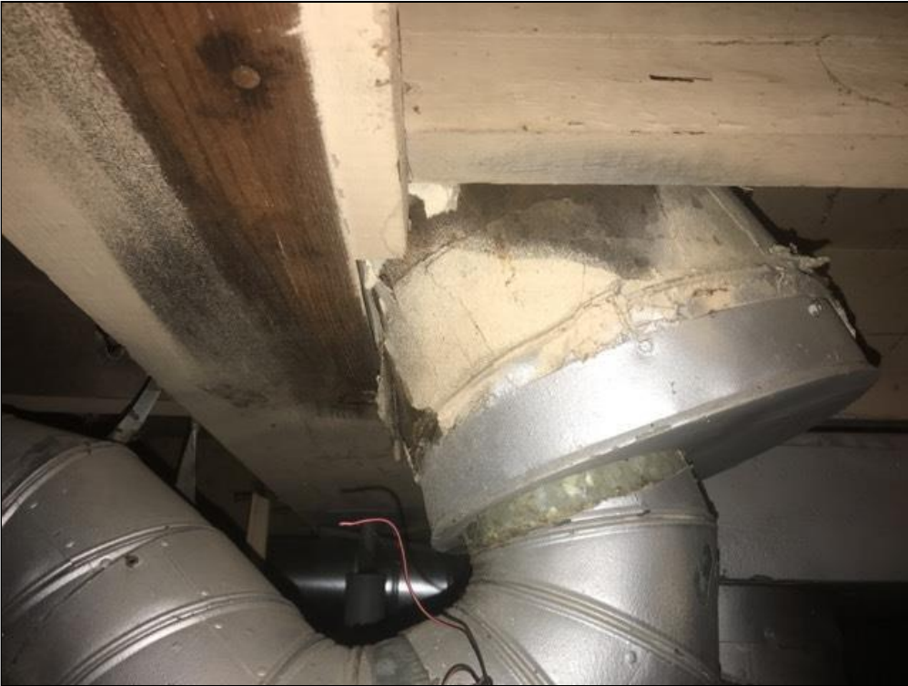
5.0 Item 7(Picture) basement hvac vent duct
