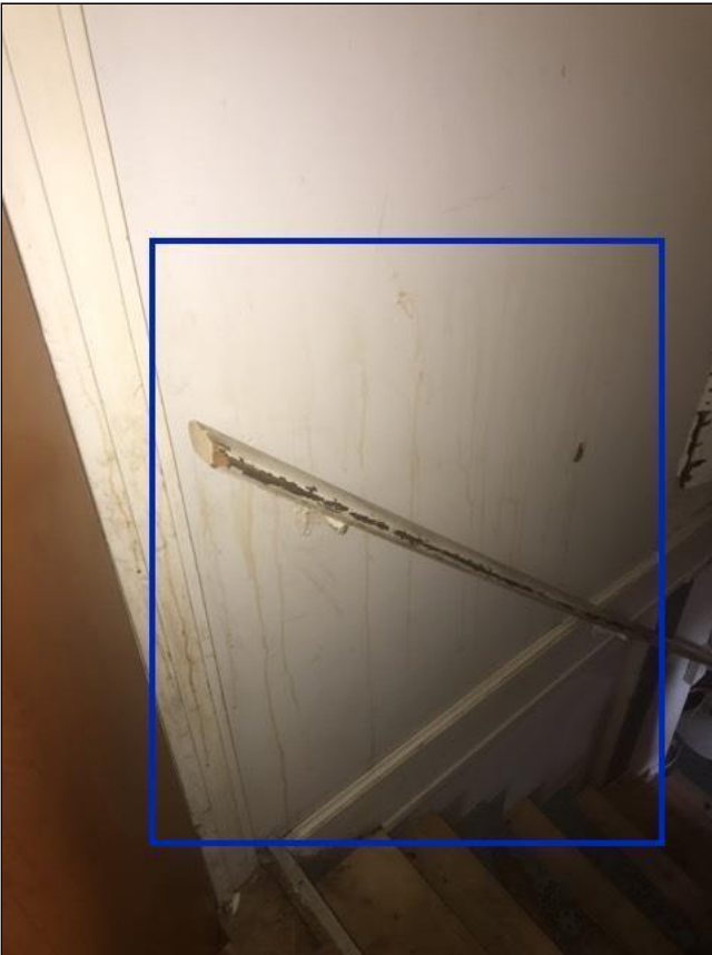
4.1 Item 3(Picture) wall to basement staining
