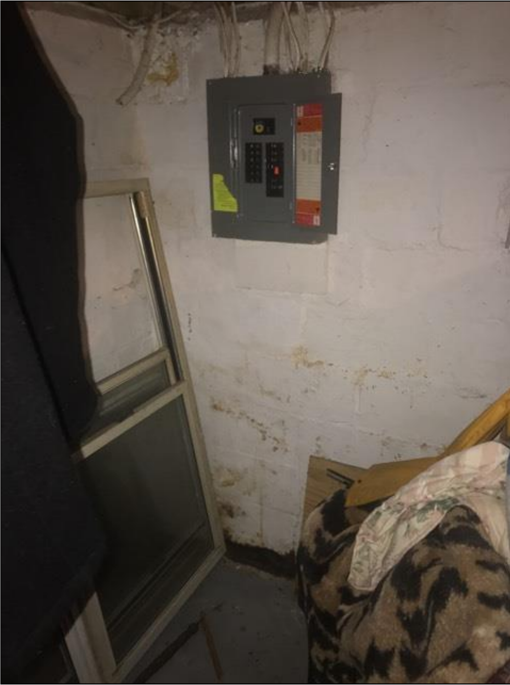
5.0 Item 6(Picture) basement wall staining
