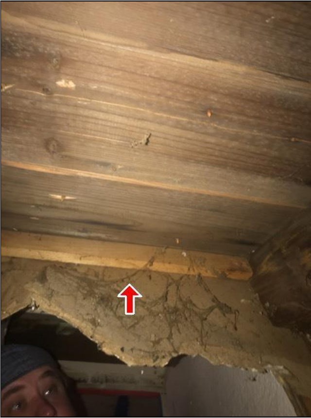
9.3 Item 2(Picture) blocked rafter cavity
